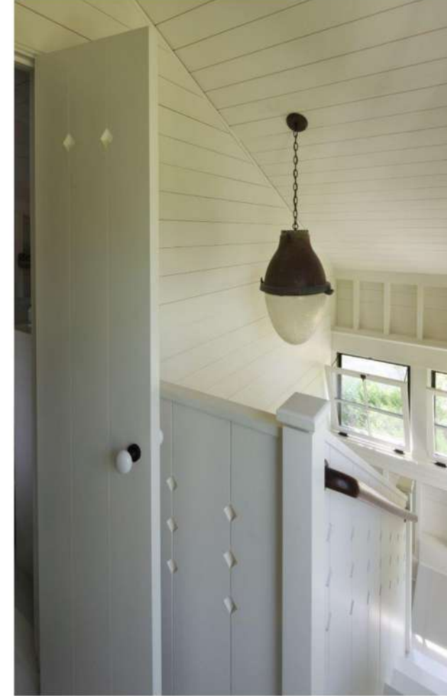
MILLWORK DETAIL VENT HOLES LINED UP WITH NICKLE GAP
